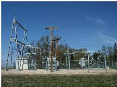
Image: Electrical substation
