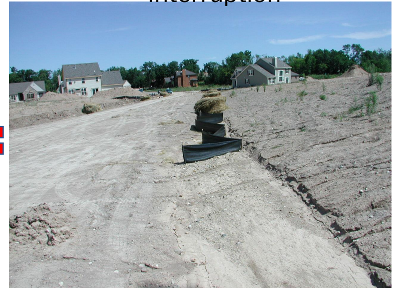
Perimeter Sediment Control & Slope Interruption
