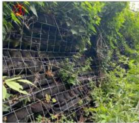
AREA OF BOWING / SLUMPING
