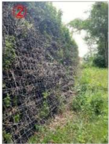
VIEW LOOKING EAST FROM EDGE OF FAILURE AREA
