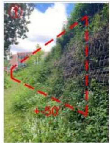
VIEW LOOKING WEST TO FAILURE AREA
