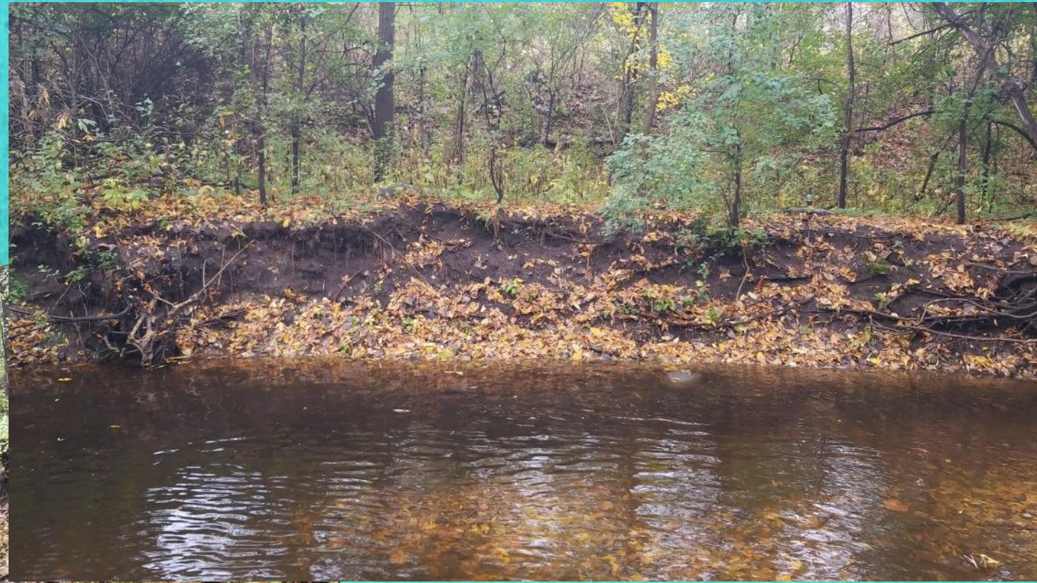
Steep failing banks
