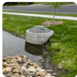
A riser pipe with trash rack
