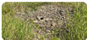
Before and after photos of vegetation management on riprap surrounding an outfall
